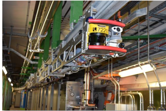
Train Inspection Monorail (CERN made)
