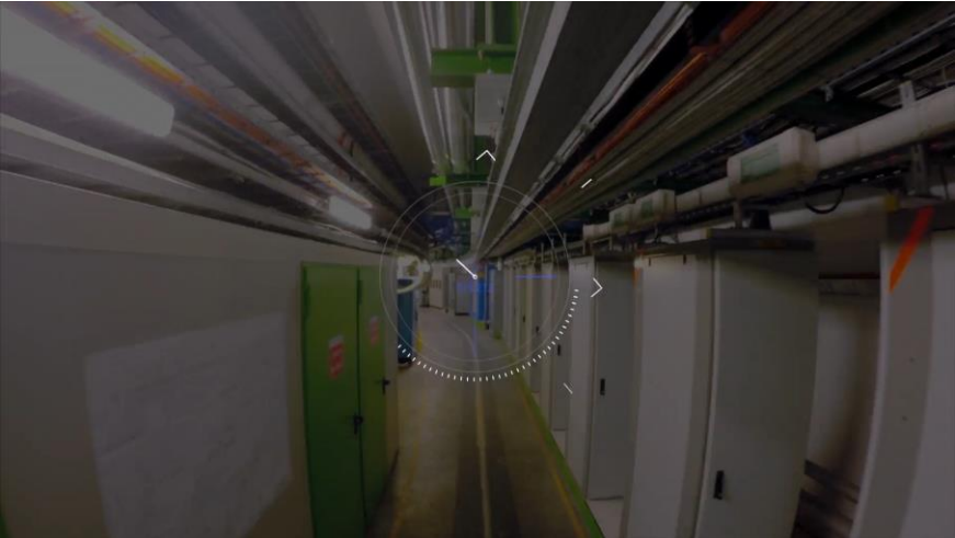
4x Train Inspection Monorail (TIM)
