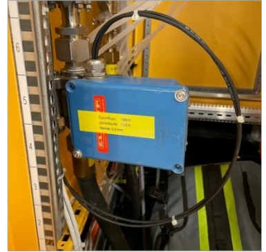
The cooling water flow-switch that generates the cooling water interlock signal.
