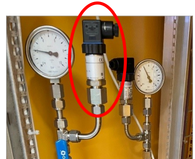
Manometers and pressure gauges to measure the pressure drop over the cooling circuit.
