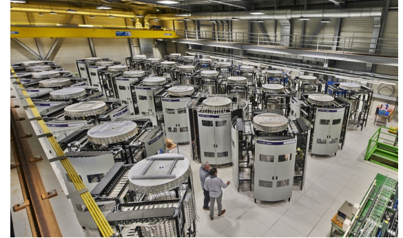
Thales 200 MHz solid state RF plant 2x 1 MW
