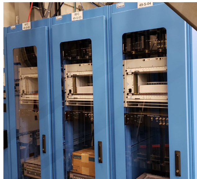
LLRF row 49 racks – Phase 2
