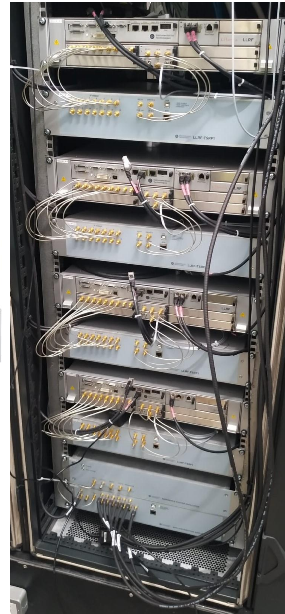
One of the four LLRF racks in DIS during pre-installation SAT period
