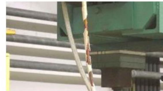
Cabling status inspection
