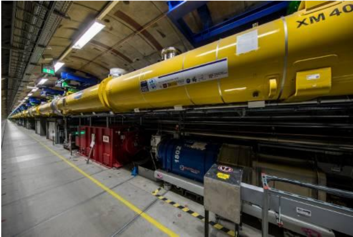
EU XFEL Linac Tunnel
