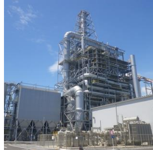
Circulating Fluidized Bed Boilers
