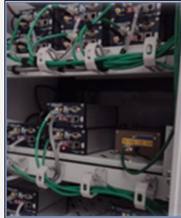
Sirius Control System nodes, for equipment control/monitor
