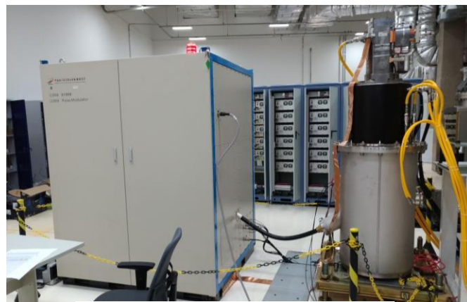
Linac Klystron and modulator
