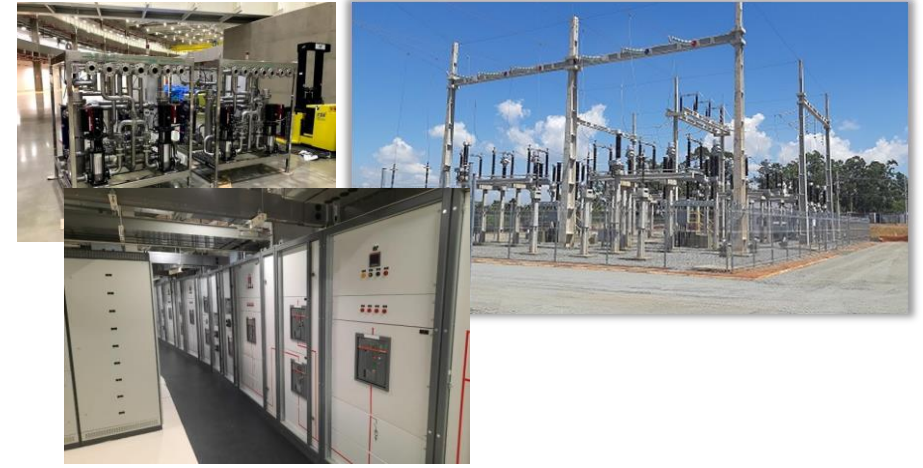
Management of CNPEM critical services (no breaks, Sirius air conditioning, etc)
