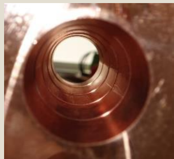
Scraper: Water pipe is embedded in Cu
