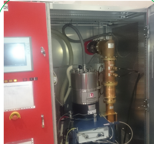
ALBA Main RF IOT based transmitters
