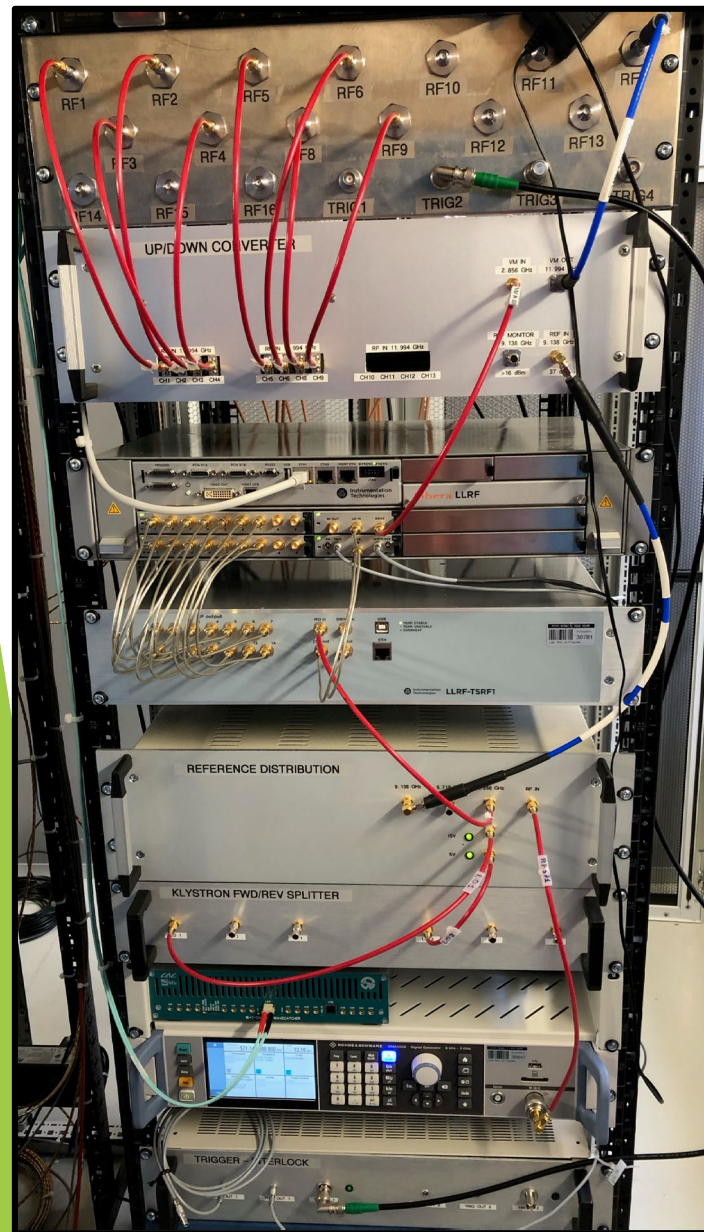
LLRF rack installed
