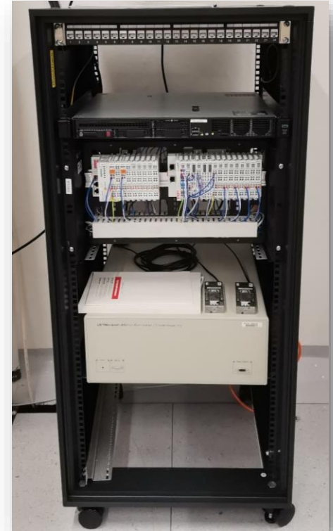
First hardware installation at the CaSIT test infrastructure / base location, courtesy of Kurt Bitterli
