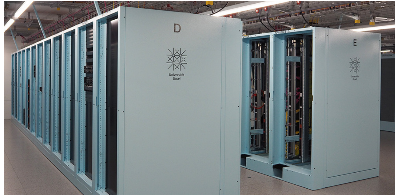
Uni Basel data center at Biozentrum
