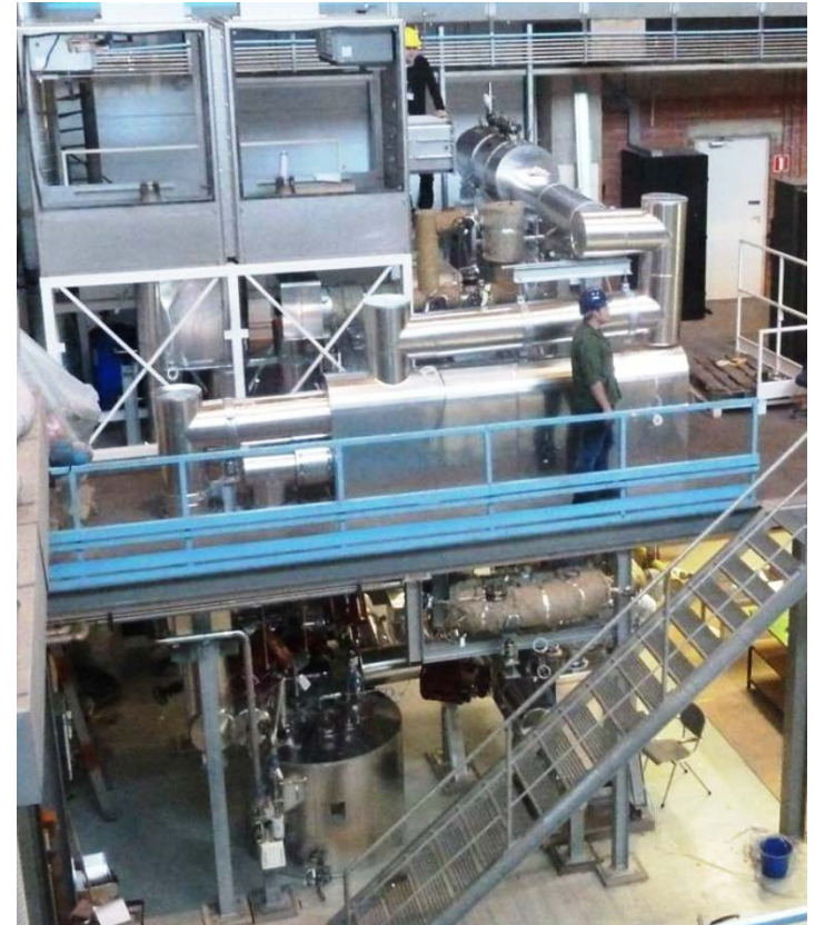
Corrosion in flowing LBE
