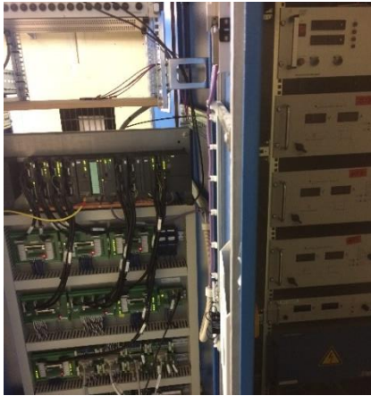
Power supply 50 kV, 200 mA
