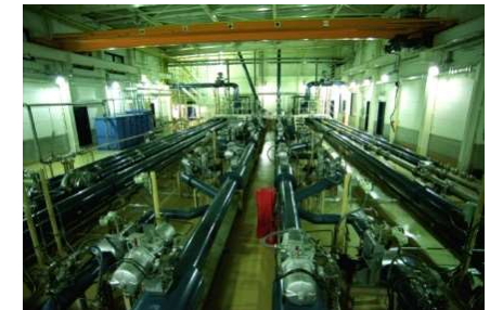
Hydrocarbon flow facility
