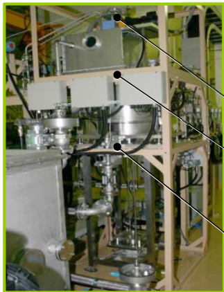
Weighing tank system
